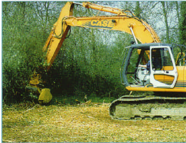
Mulching under electric lines
